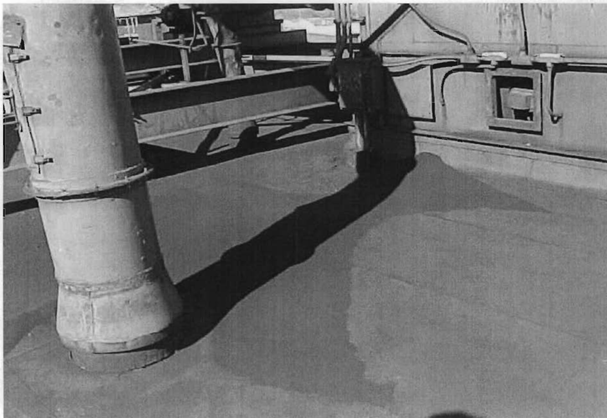
4. Facility Roof before BMPs. Dust accumulation on facility roof.
