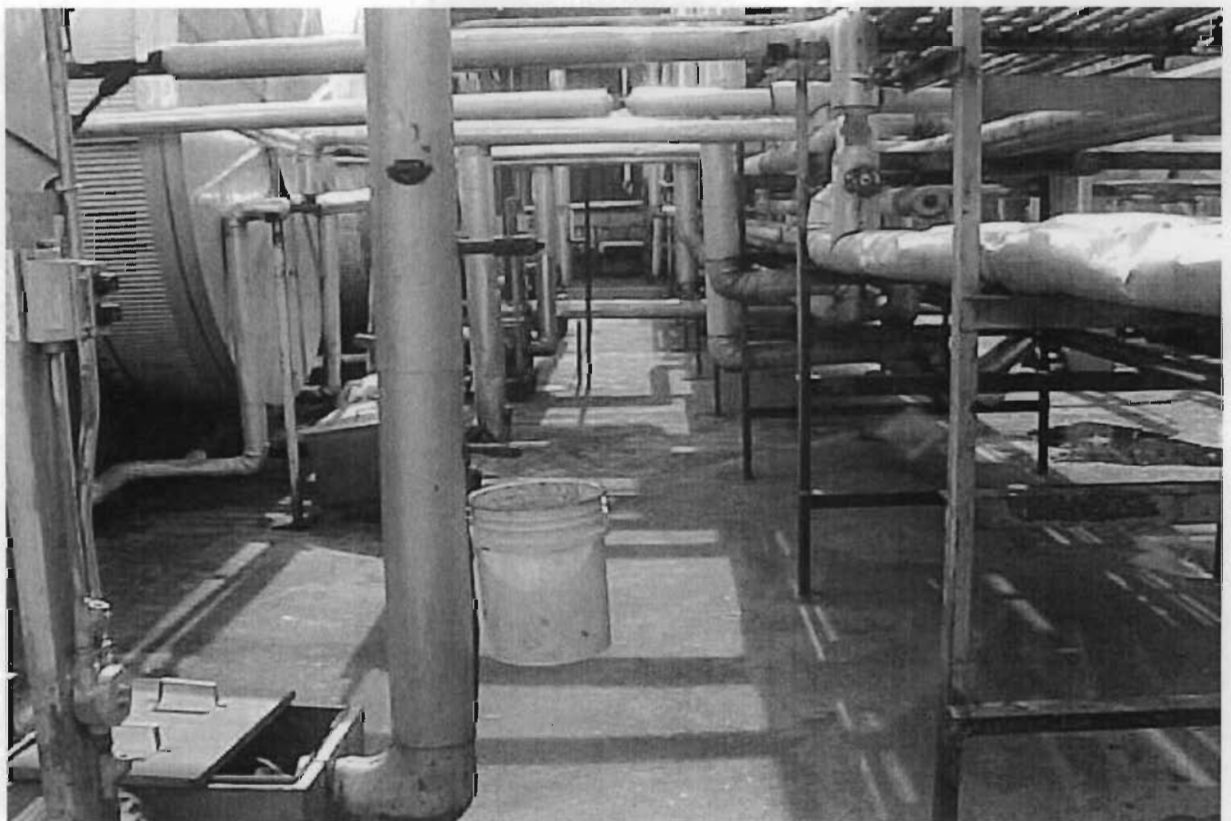
13. Tank Farm after BMPs. Pumps serviced to prevent leaks, covered to prevent exposure, daily inspections.
