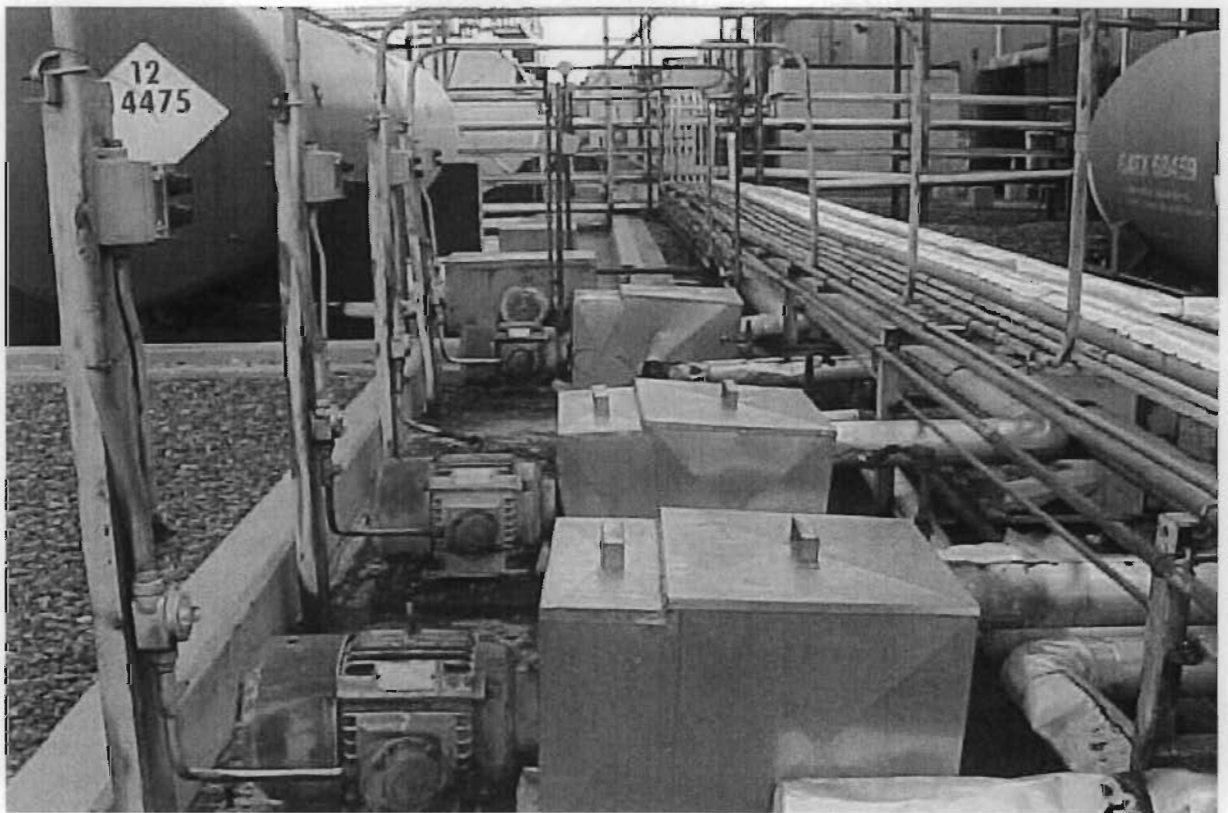
15. Tank Farm after BMPs. Pumps serviced to prevent leaks, covered to prevent exposure, daily inspections.
