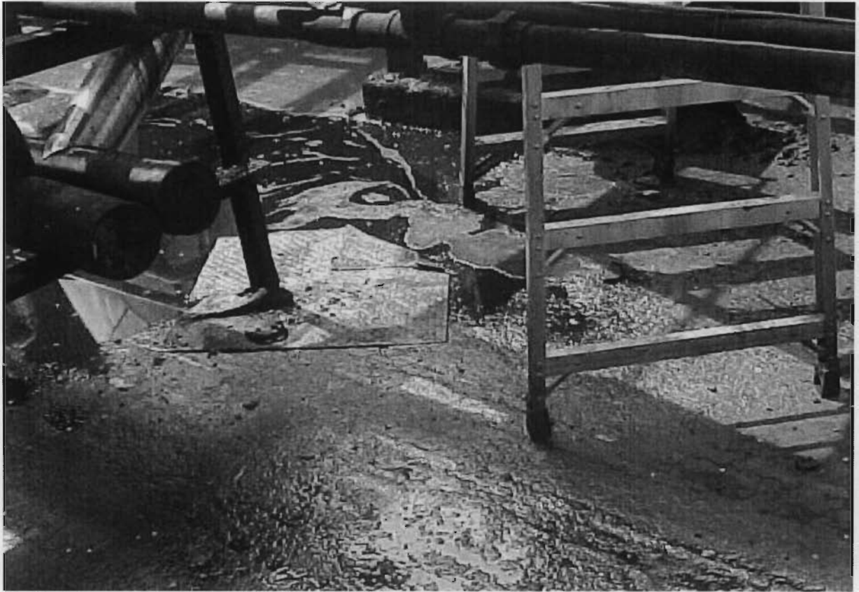
14. Tank Farm prior to BMPs. Oil leaks potential stormwater exposure.
