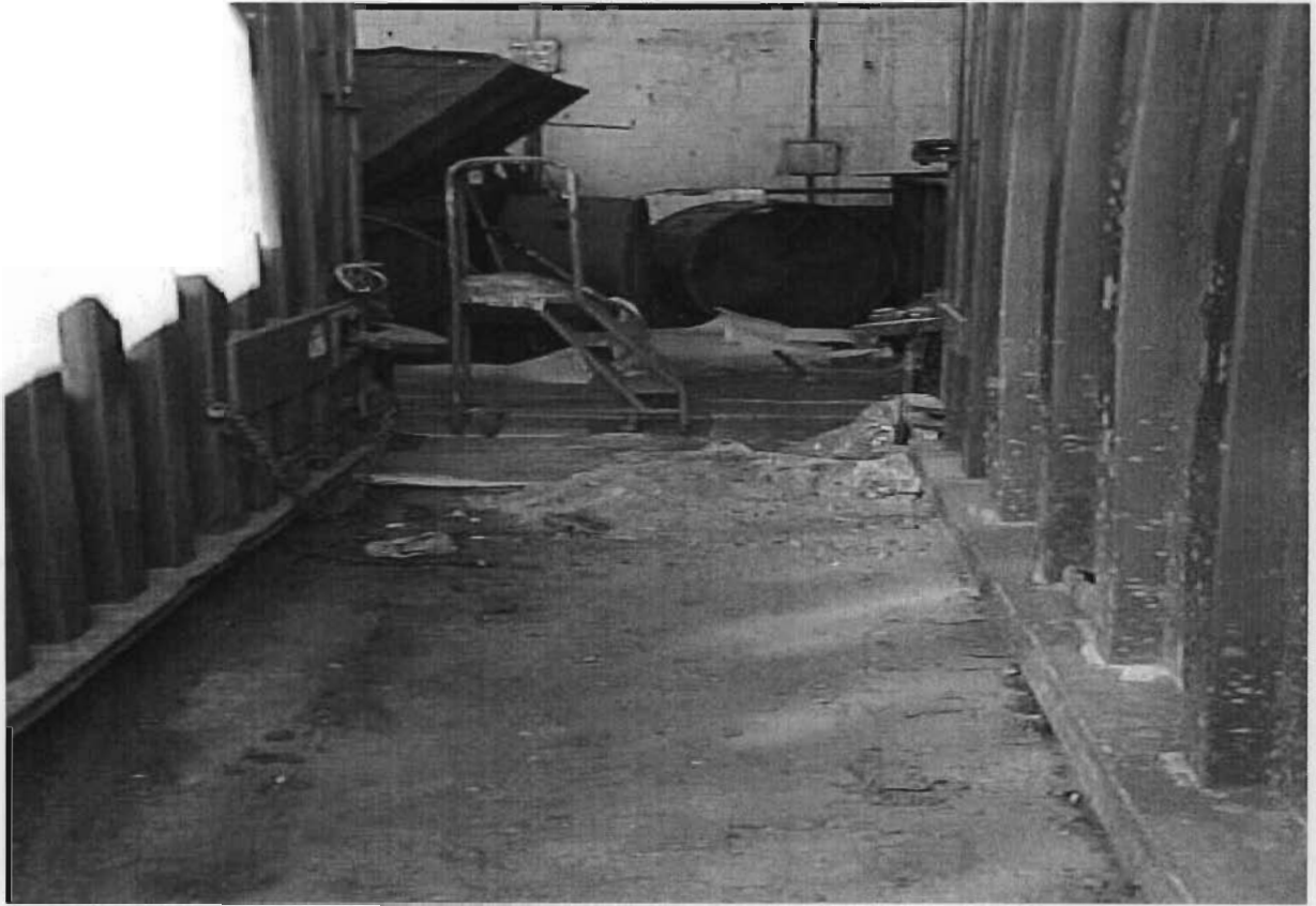
7. South Waste Compactor Area prior to BMPs. Dust and Waste potential exposure to stormwater.
